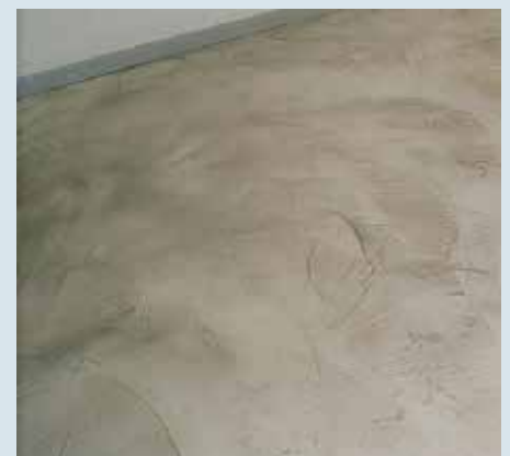
OLD EPOXY OR POLYURETHANE COATINGS
